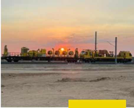
HIGH SPEED LINE- Egypt Commissioning of a Vehicle Set for the Electrification of the High-Speed Rail 'HSR Green Line'
