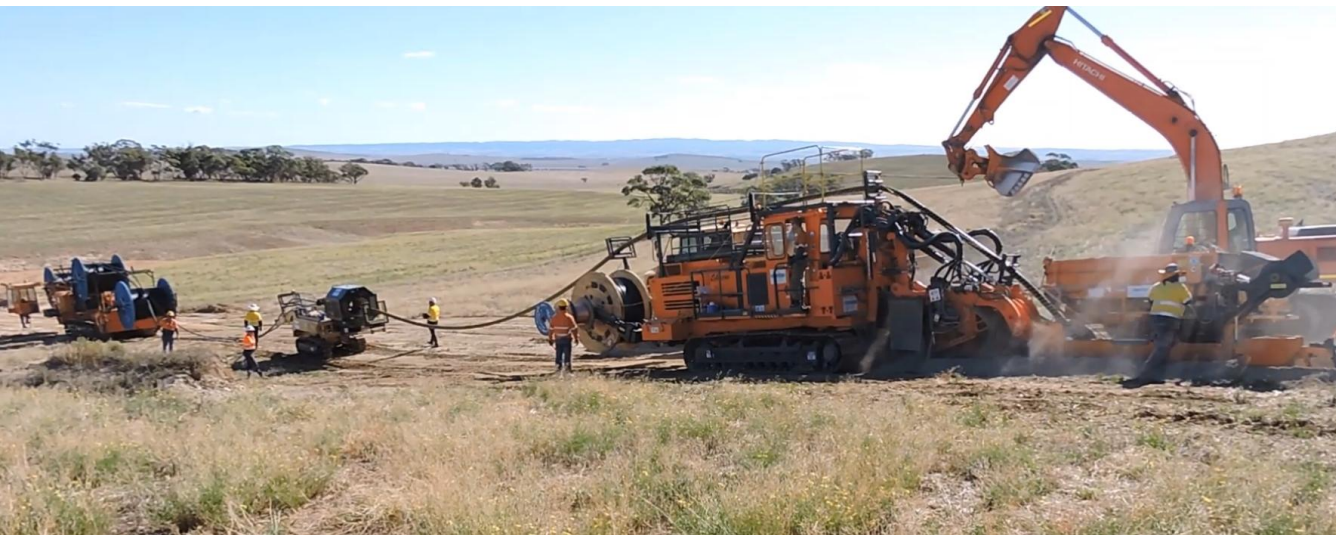
Smart, green and cost savings working system
